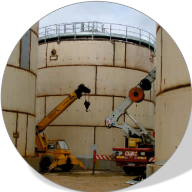
Storage tanks EMIT Construction of storage tanks at the central gas turbine Scandale (KR). Customer: E.M.I.T. S.p.A. Year : 2007
