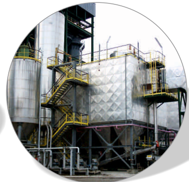
Filters Hamon sleeves Prefabrication and assembly of bag filters. Commissioned Hamon Research Cottrell. End customer: Biomass Italy. Year: 2001
