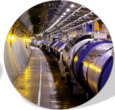
Piping LHC tunnel at CERN Piping installation in the LHC tunnel at CERN in Geneva. Work commissioned by the Renco S.p.A. and executed in 2002.
