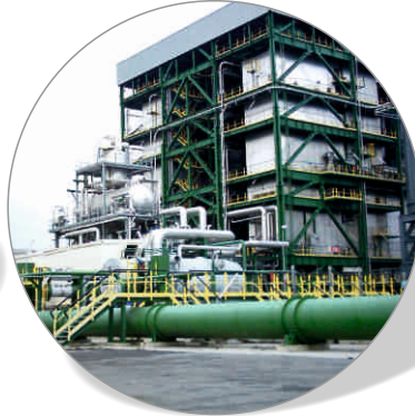
Central carpentry biomass Construction and installation auxiliary carpentry. Work done in workshop O.M.G. Strongoli (KR) in 2001, Gallo S.p.A.
