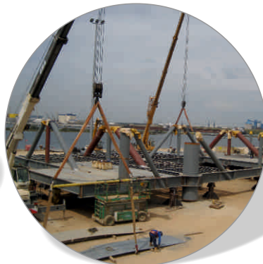
Deck West Franklin and Elgin B Prefabrication and assembly sub assembly deck West Franklin and Elgin B, at the Shipyard Piomboni of Ravenna. Customer: Rosetti Marino S.p.A. | 2012
